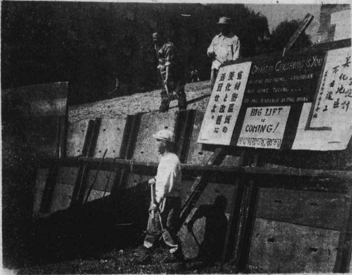
These Seattle JA CLers are among many residents of the Jackson St. area who turned out recently for the first Sunday operation of "Big Lift", a community improvement project to landscape a steep empty lot. Topping are Arthur L. Solomon, Jr., head worker of Neighborhood House, and Tak Kubota, noted landscape contractor who has charge of some 800 trees and shrubs. Below is Dr. T. T. Nakamura, dentist, about to heave a shovel into the truck. Sign proclaims "Big Lift" in five languages: English, Hebrew, Chinese, Japanese and Filipino. —Elmer Ogawa Photo.
