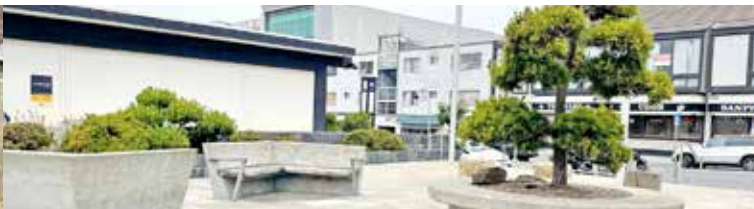
Casual and informal seating in Peace Plaza; numerous pavement stones have been cracked through the years, some by illegal skateboarding.
